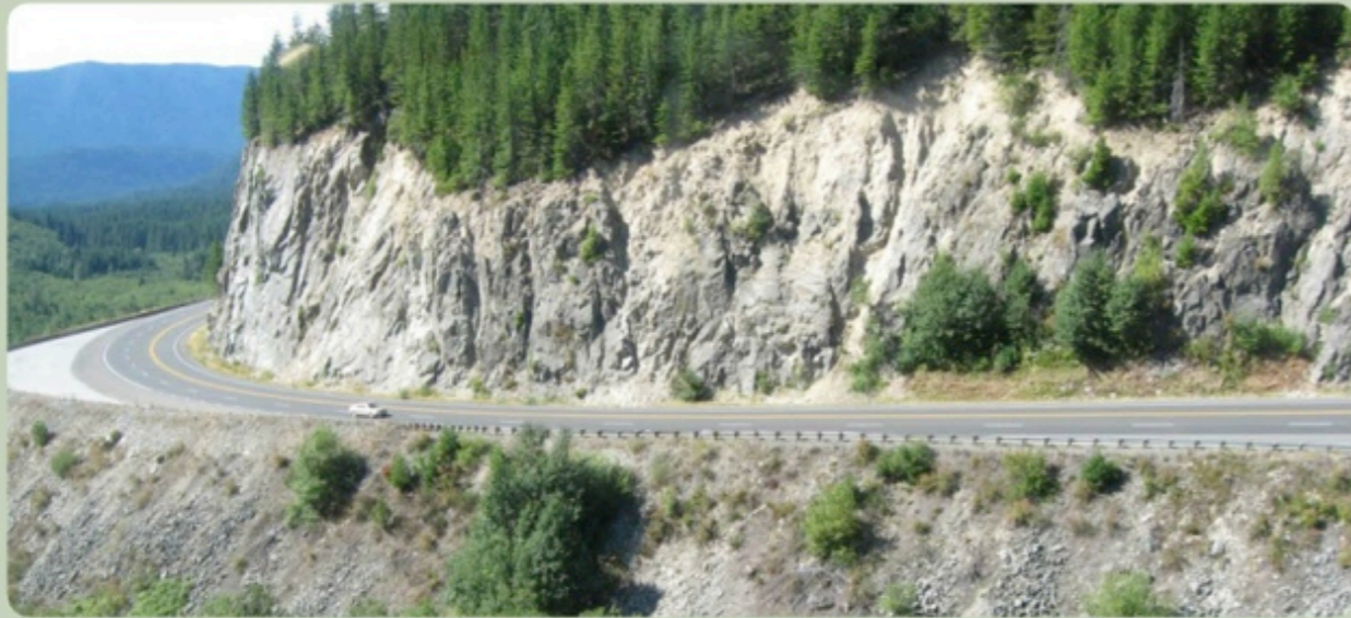
ODOT is looking to cut the rock slope back from the roadway and design a more stable rock slope
