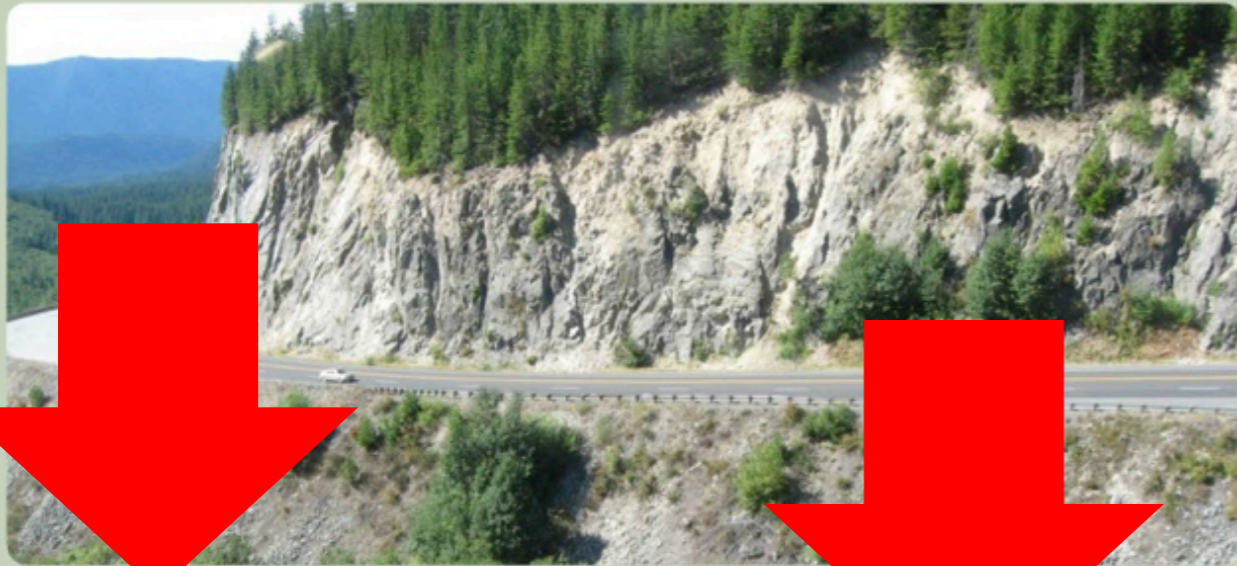
ODOT is looking to cut the rock slope back from the road to create a more stable rock slope
